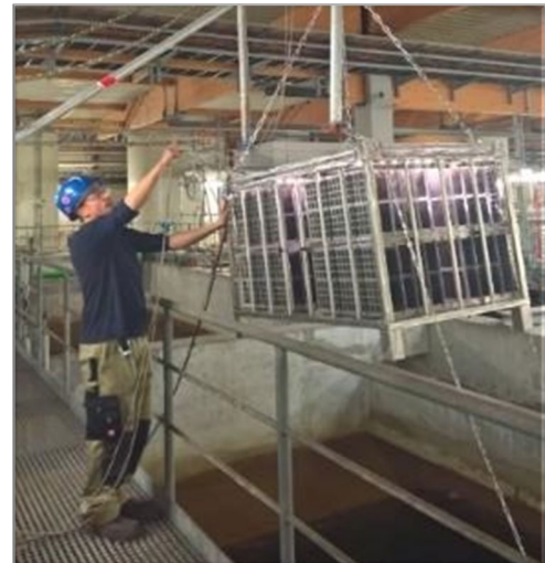
Figure 3: Catalytic module in the treatment of fresh water at the Schkopau power station
